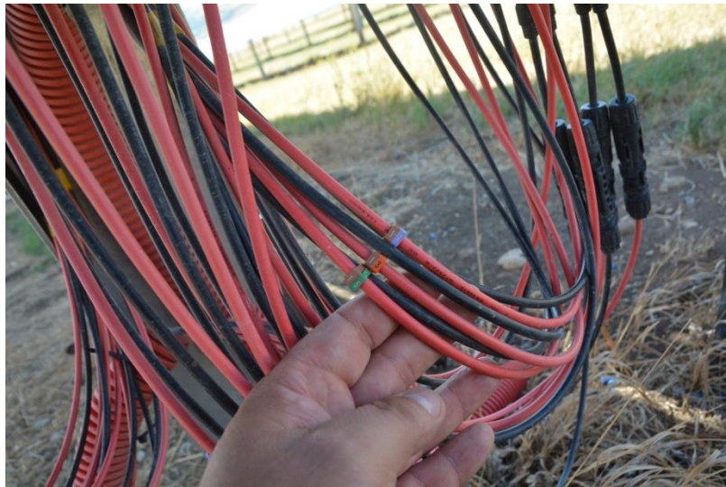
DC cable labeling
