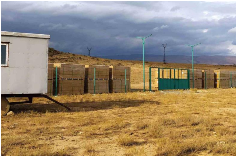
Fencing and gate is provided for laydown area
