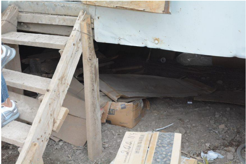
Construction debris left uncleared
