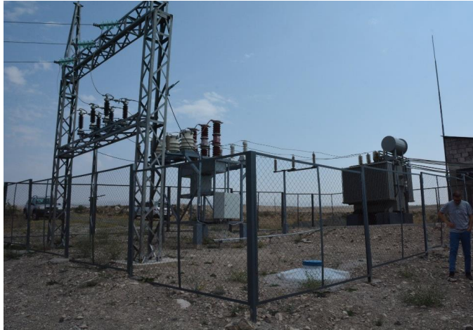
Substation fencing following local regulation
