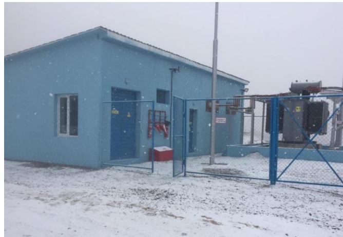
Substation fencing should be lockable
