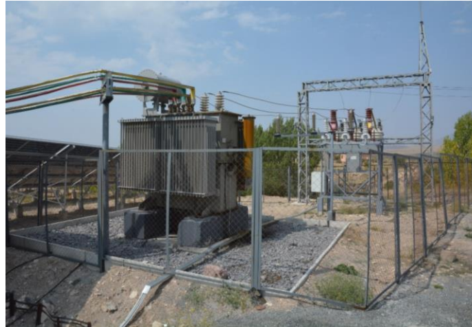
Substation fencing following local regulation
